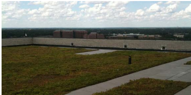
Ford World Headquarters Green Roof – Dearborn, Michigan
