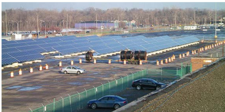
The Michigan Assembly Plant – which produces the Focus Electric, C MAX Energi, C MAX Hybrid and gas-powered Ford Focus – is powered by one of the largest solar arrays in the state of Michigan.
