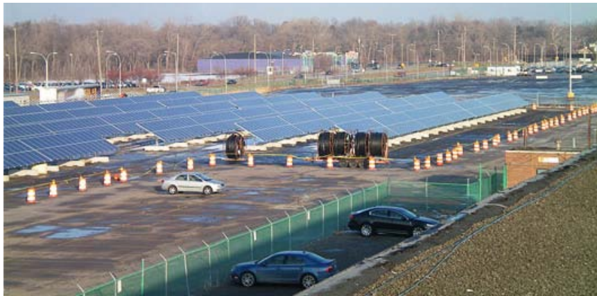
The Michigan Assembly Plant – which produces the Focus Electric, C-MAX Energi, C-MAX Hybrid and gas-powered Ford Focus – is powered by one of the largest solar arrays in the state of Michigan.
